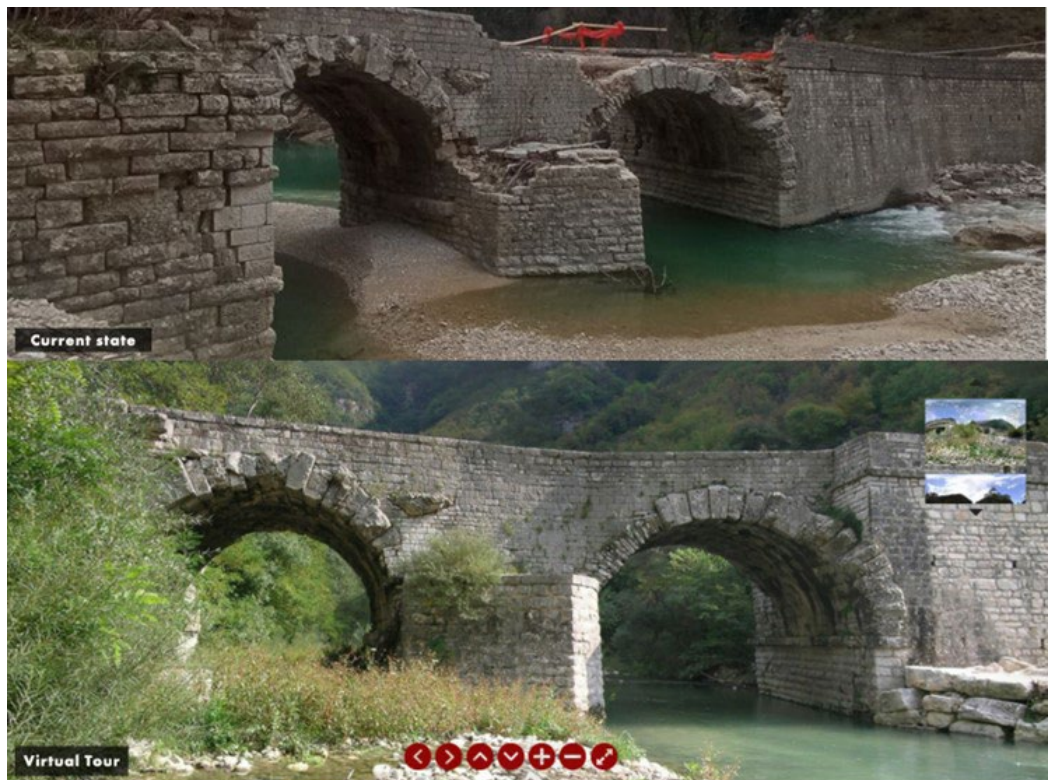
Fig. 4. Top, the current state of the Ponte Grosso in Cantiano (PU) after the alluvium's damages. Bottom, a scene from the bridge's Virtual Tour from the DCE website.
