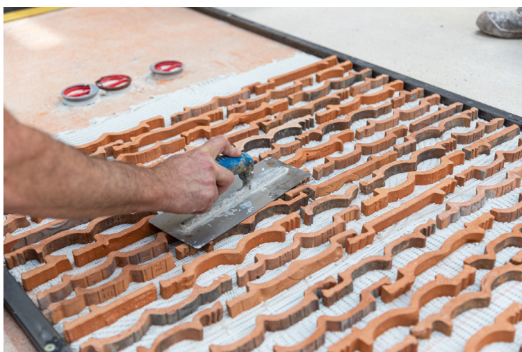
Fig. 5 - Detail of the floor construction with recycled roof tiles at the building site of Le Magasin Électrique, LUMA Arles, France (Image courtesy of © LUMA Arles, ph. Credit © Adrian Deweerdt)
