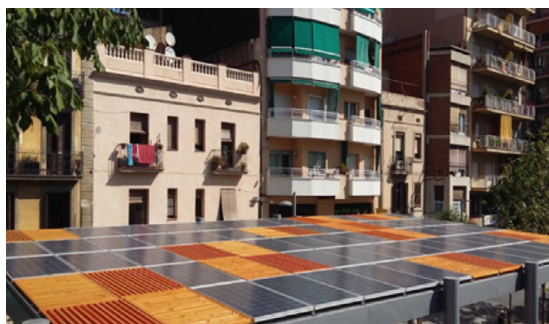
a. Photovoltaic pergola over a children's play area in Barcelona's Plaça del Centre.
