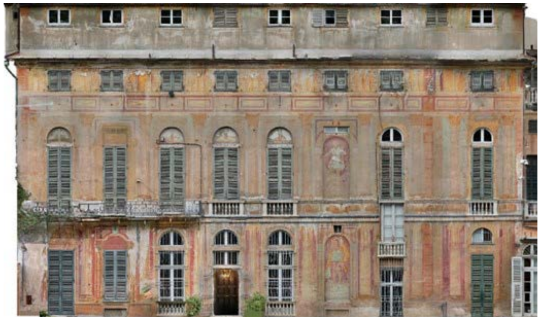
Fig. 9. Aerial photogrammetric survey by drone of the secondary façade overlooking the garden. Elaboration by the authors.
