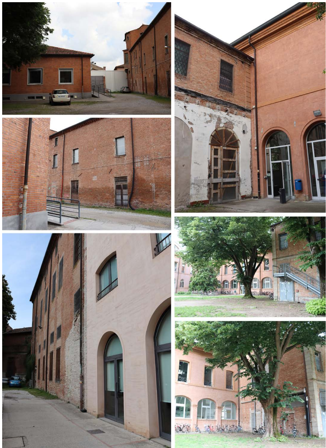
Fig. 3. Views of Palazzo Tassoni Estense, highlighting the parts currently in use and those in need of restoration. Photos by the authors.
