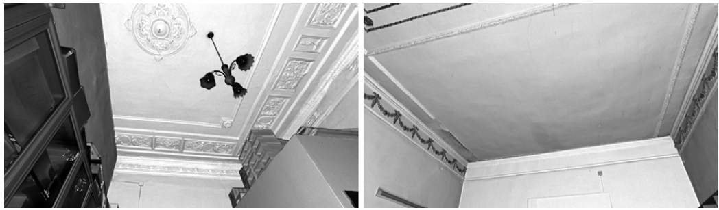
Fig. 9. Stucco decorations of the ground floor interrupted by the introduction of more recent construction. Points cloud model views. Elaboration by CHM_lab.
