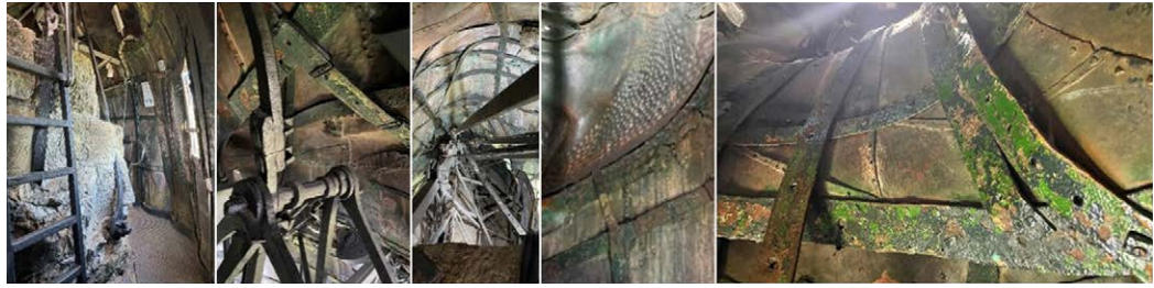
Fig. 3. Some overview and detail photos of the interior of the head, highlighting the metal support structure of the "cage" to which the copper plates are anchored. Elaboration by the authors.
