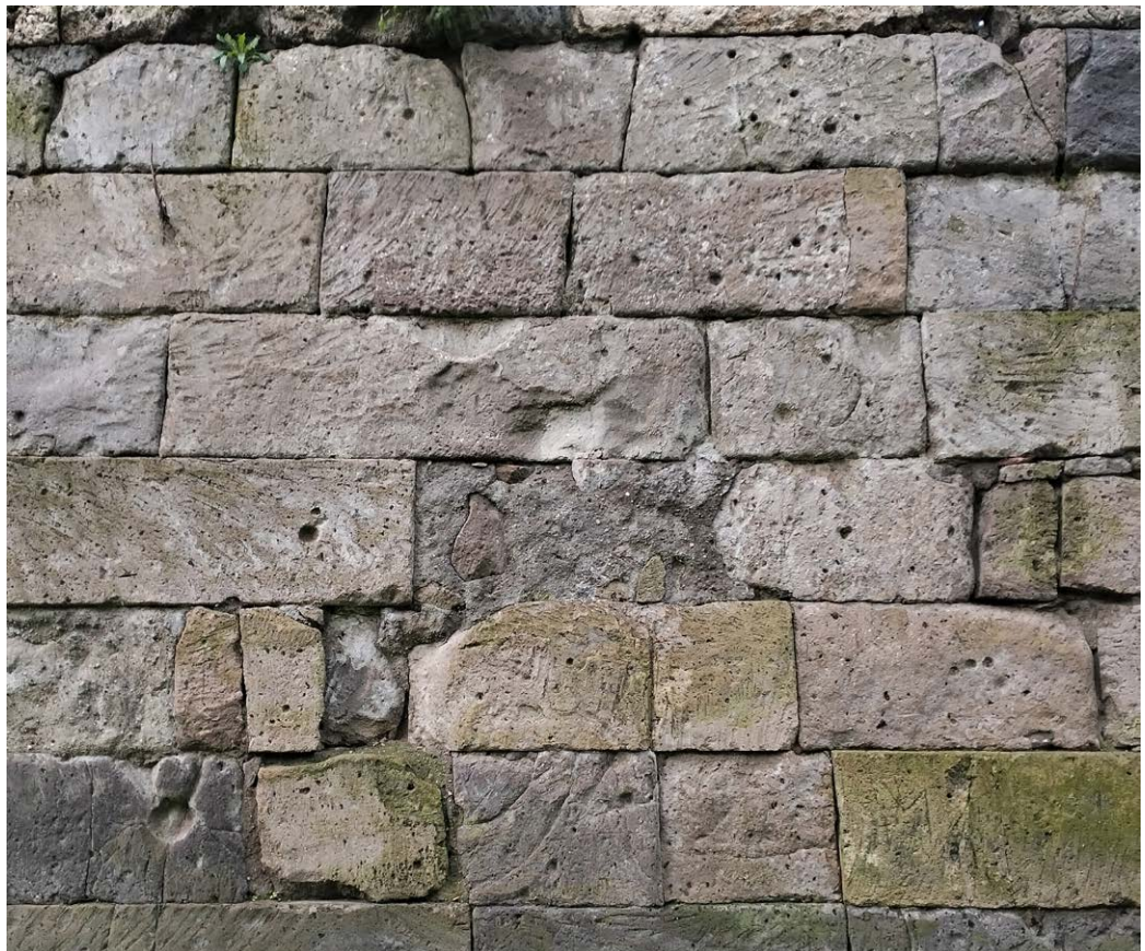
Fig. 1. Section of the ancient city walls chosen to demonstrate the methodology. Image by the authors
