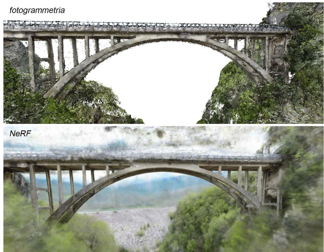
Fig. 8. Arcichiaro Bridge: visual comparison between the photogrammetric textured model and NeRF volumetric rendering. Elaboration by the authors.
