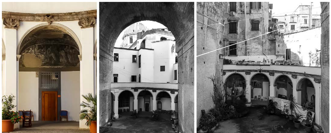
Fig. 3. The lower cloister, oval in shape, violently compromised by the invasion of the piers of the Corso Napoleone Bridge, now Ponte Maddalena Cerasuolo. Photo by I. Izzo, 2018.
