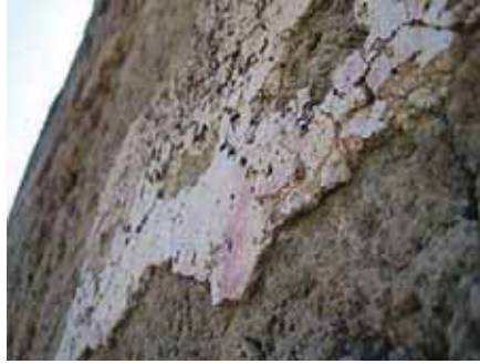
Fig. 06 : Santa Maria in Campogrosso, detail of the plaster in the inner part of the masonry of the central apse
