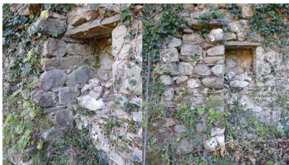
Fig. 07 : Wall H where - on the side of one of the niches - one can see a contemporary perpendicular wall, later cut
