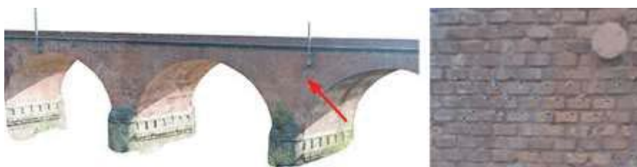
Fig. 04 : Case C. Tiled view of Mereta I bridge 3D model and marked bricks
