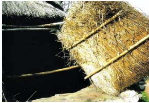
Fig. 11 : Mealha, Tavira: boqueirão opened on the cover, made to place the straw inside (Almeida, 2010, p. 86)
