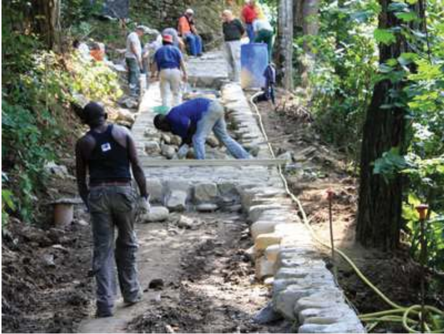
Fig. 01 : San Piero in Bagno (FC)_ Italy. The work of volunteers of Faro di Corzano Association for the reconstruction of a medieval mule road (CORNIETI 2012)
