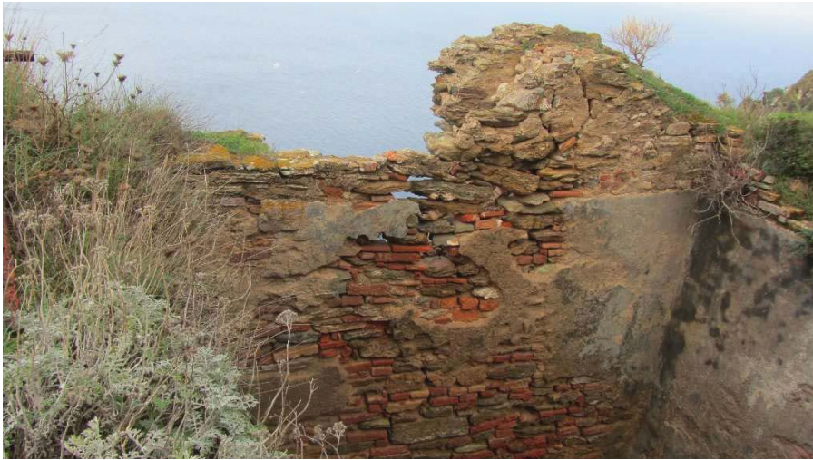
Fig. 10 : "Sack" wall in the phase of collapse and weeds vegetation (photo by authors)
