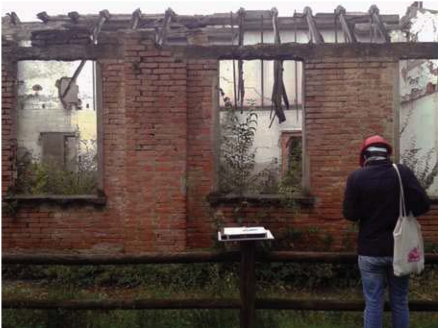
Fig. 02 : Ex Fossoli Camp, Carpi (MO)_ Italy. A voluntary worker during inspections for conservation program of ruins of building for prisoners (UGOLINI 2011)
