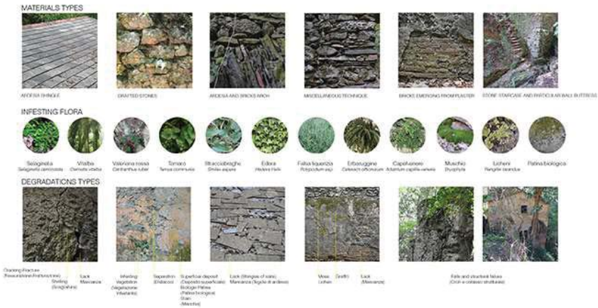
Fig. 04 : List of material, infesting flora and deterioration types, all noticed during the survey campaign (for the infesting flora see also the reference OLIVARI, ROTTA (1988) - I mulini dell'Acquaviva sul Monte di Portofino , Sagep Editrice, Genova
