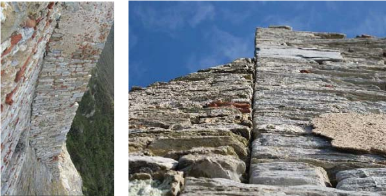
Fig. 03 : Wall on the rock(photo by the authors). Fig. 04 : Successive phases of construction (photo by the authors)
