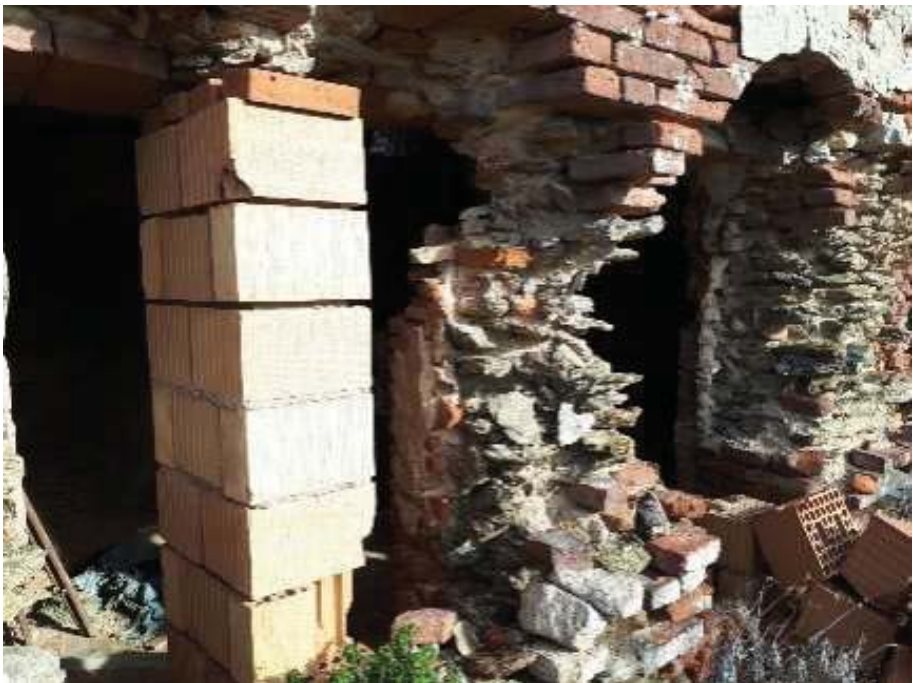
Fig. 09 : Decay phenomena and urgencies interventions (photo by authors)
