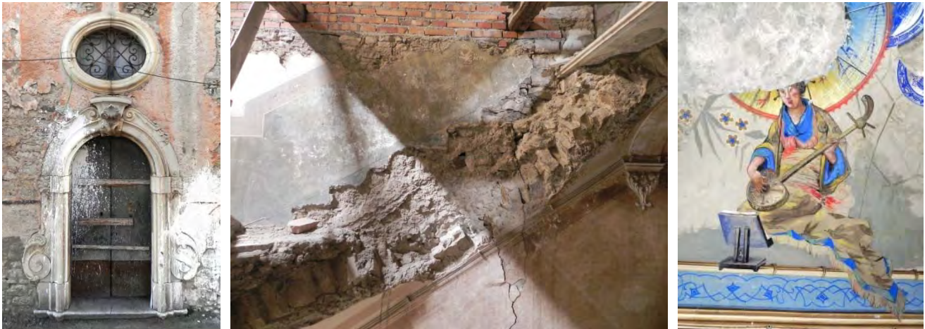
Fig. 4 – On the left: stone baroque portal. In the middle: remains of the collapsed terminal flight of the internal masonry vaulted staircase. On the right: Detail of the wallpainted Chinese room
