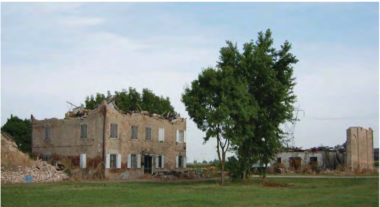
Fig. 1 – San Giacomo Roncole in the district of Mirandola (MO), in the historic courtyard the stable-barn and the dwelling collapsed due to wall-roof interaction.
