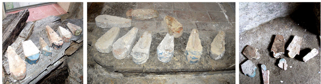
Fig. 2. Sicily, shaped wedges: up, three-dimensional reconstructions of some of the most frequent cases; down, examples of wedge-shaped bricks used in the same spire with different tapering angles.
