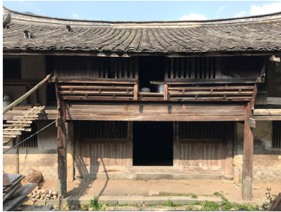
Fig. 3. Front view of the access system to the distribution galleries (photo by M. Calia, March 2019).
