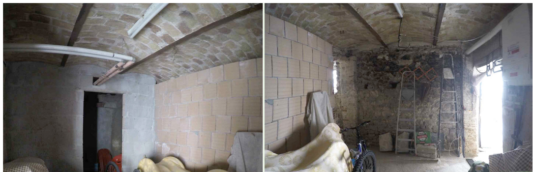
Fig. 8. Brick vaults of a building in the historic centre of Castel del Monte (AQ), (photo by V. Cetra).
