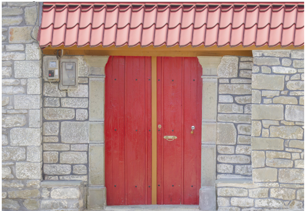
Fig. 9. Traditional roof cover replaced with plastic elements.
