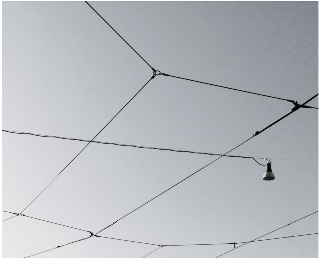
Fig. 3. Electric tram cables, as components and connection signs.
